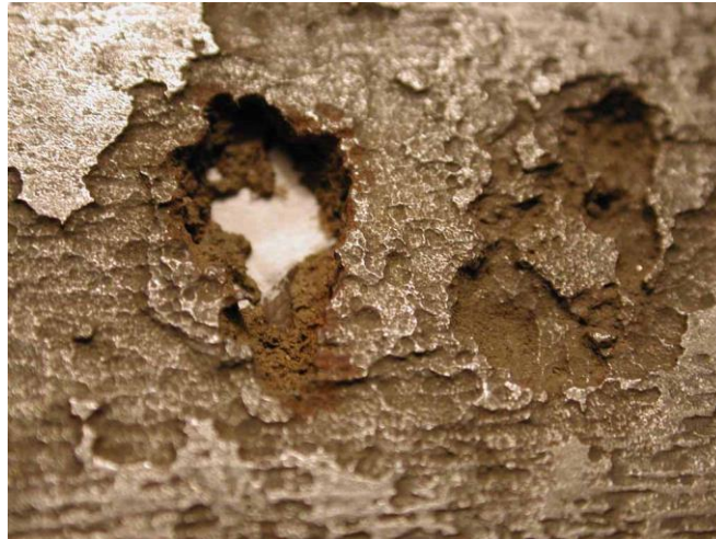
Corrosion of a heating oil tank by Sulphate Reducing Bacteria (SRB)
